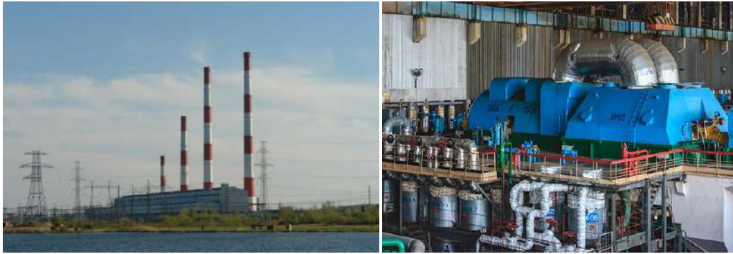
Figure 2. View of the main building from the side of the engine room of Zainskaya SDPP (a), view of the engine room inside Zainskaya SDPP (b)
