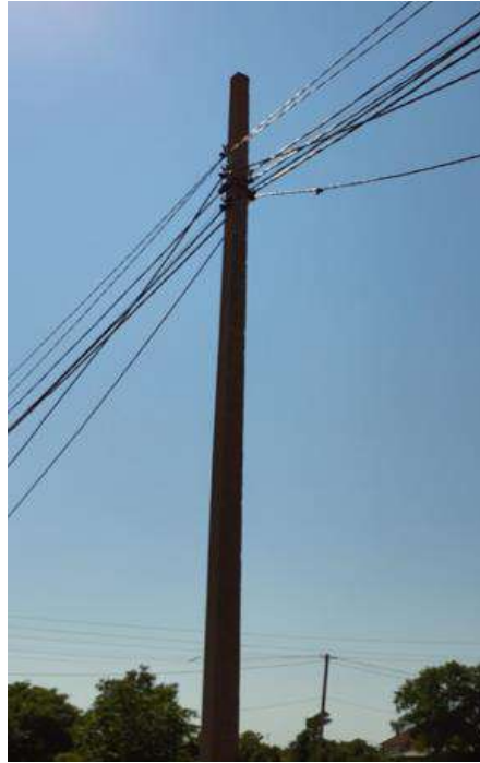
Figure 1. Location of six overhead lines on the support
