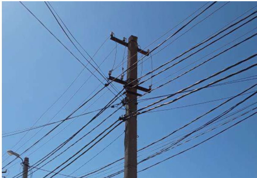
Figure 5. Passage of several overhead lines by joint suspension, including uninsulated
